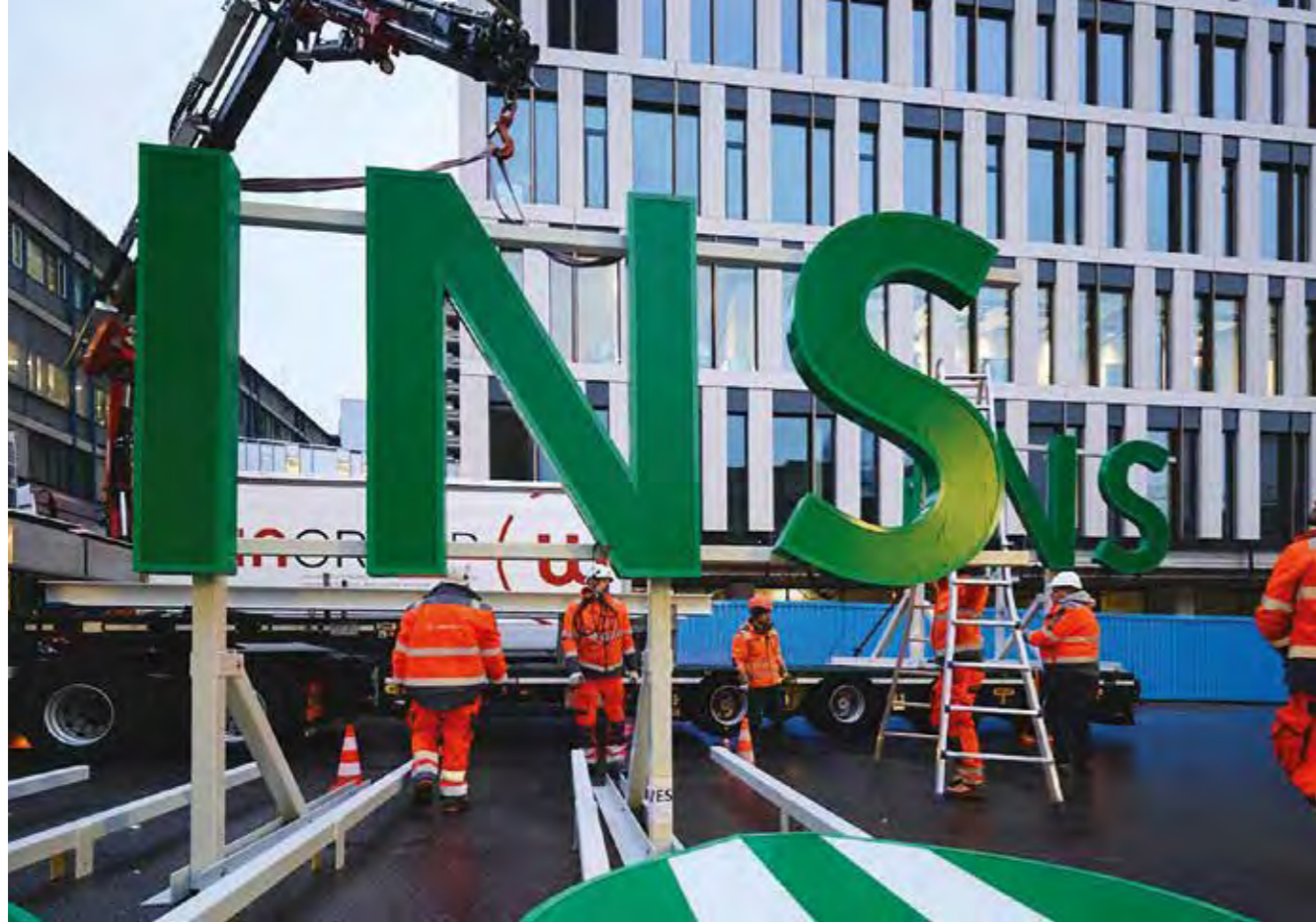
The future centerpiece of the Insel-Campus becomes visible in 2022: The "Insel"-letterings were installed on the new main building Anna-Seiler-Haus at the end of November 2022.
